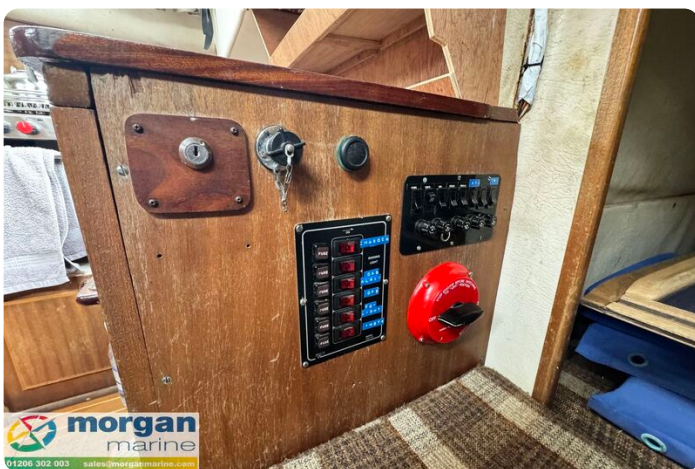
Westerly Griffon MK1 - switch panel
