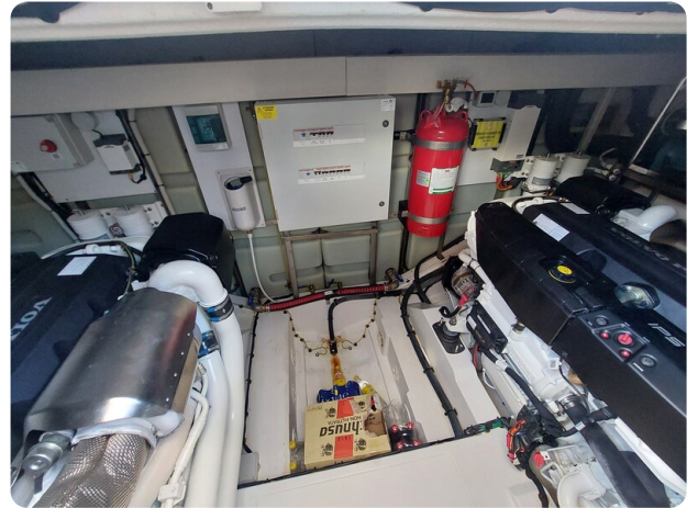
Azimut 53 Fly engine room
