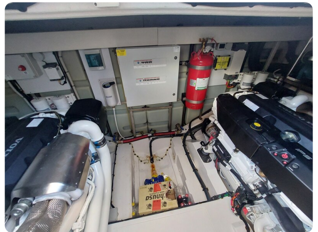
Azimut 53 Fly engine room
